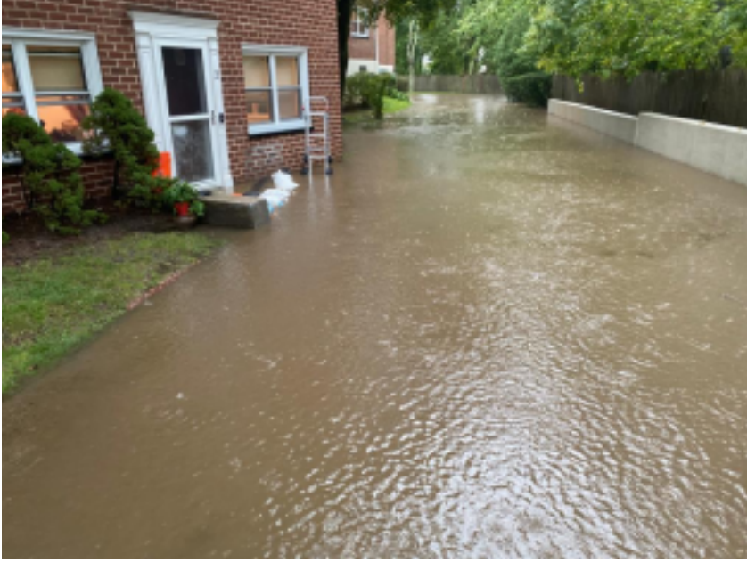
- Entrance to 2 Charter Circle from 9/29/23 rainstorm.
